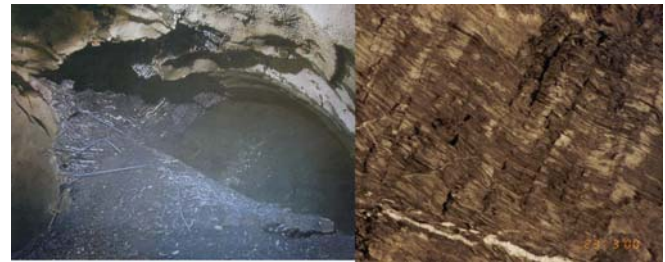
Figure 5. Headrace tunnel collapse at Kali Gandaki 'A' Hydroelectric Project (left) and tunnel face showing thin foliation plane with very weak bond (right) (Panthi 2006)
