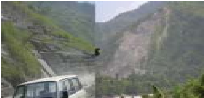
Figure 2. A major slide at Krishnabir along the Prithvi Highway, 'A main gateway to Kathmandu Valley'. Slope protection works with gabion (left) and the extent of slope failure (right)
