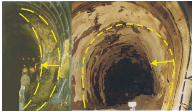
Figure 8. Severe squeezing at Modi pressure tunnel (left) and Kali Gandaki headrace tunnel (right) (Photo: Himal Hydro 2001 and Impregilo SpA 1989)
