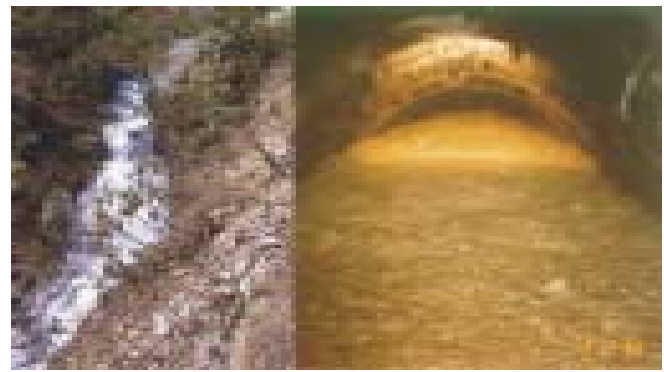
Figure 9. Water leakage from adit 2 of Khimti headrace tunnel after early water filling (left) and mass inflow of water mixed with debris from a shear fault at the pressure tunnel of Modi Khola (right) (right photo: Himal Hydro 1998)
